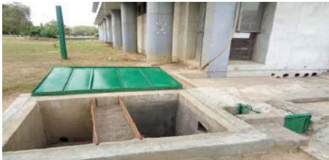
Fig. 2. Rooftop water harvesting unit for groundwater recharge
