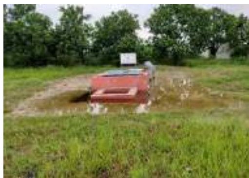
Fig. 2. Groundwater recharge cum drainage unit draining waterlogged land after monsoon
