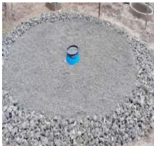
Fig. 2. Field view of installed horizontal flow filter
