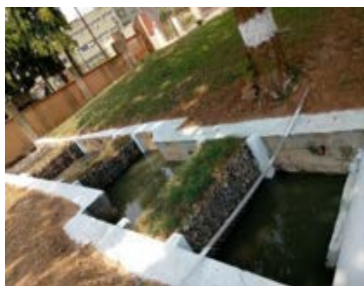
Installed wastewater treatment system
